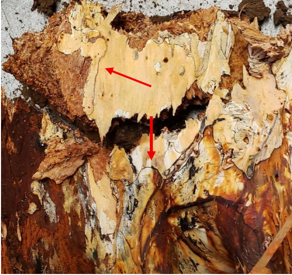
Spongy advanced decay with black zone lines
