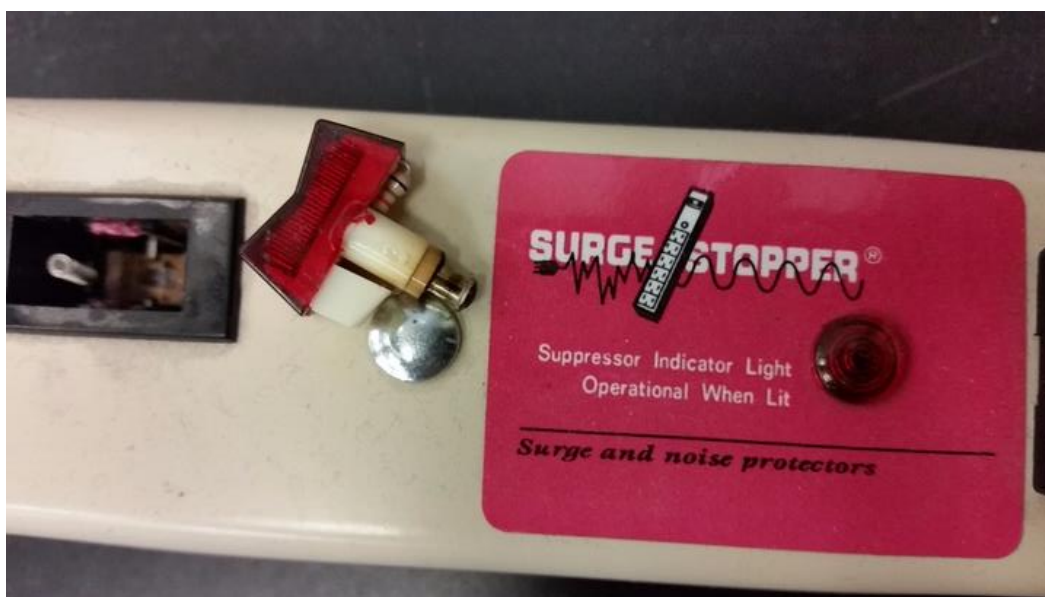
The broken switch, as documented by Carl. Notice the broken plastic on the switch and remaining in the switch housing.
