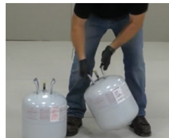
Shaking of A-side and B-side tanks
