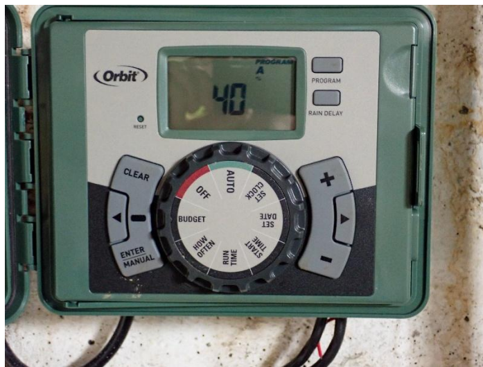
Figure 8. Automatic sprinkler controller shown with an adjusted run time of 40%, here called the “Budget” setting. Photo: A. McGuire.
