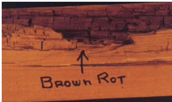
Figure 4. The final stage of wood decay by the brown rots can be identified by the dark brown color of the wood, excessive wood shrinkage, cross-grain cracking, and the ease with which the dry wood substance can be crushed to powder. Photo by: Gary Thomasson.
