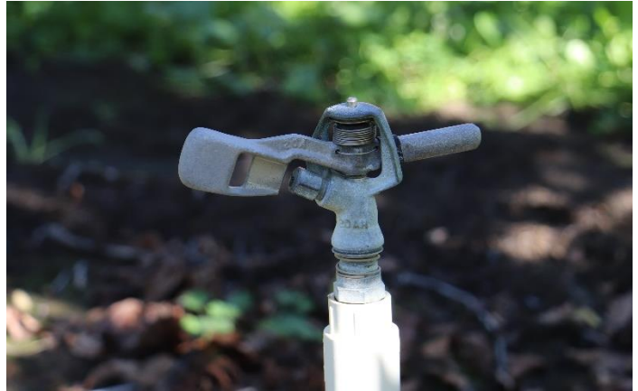
Figure 21. Rainbird sprinklers (pictured) and R2000 sprinklers were standard at this site.
