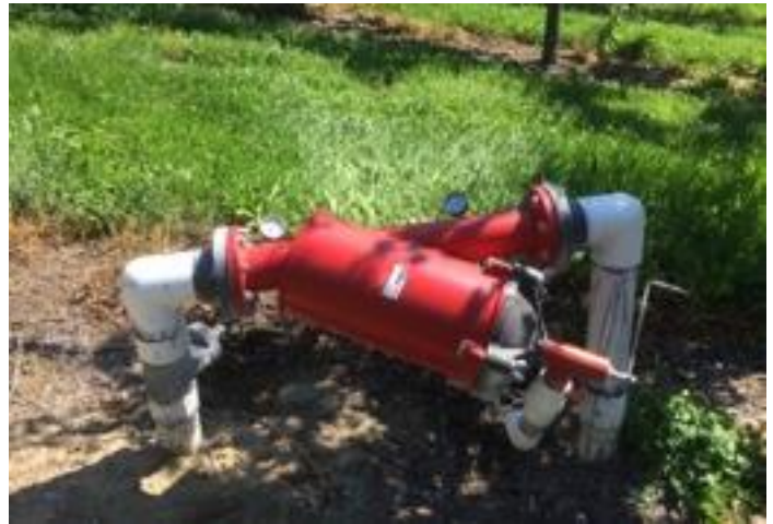
Figure 31. Brush filter can be cleaned by turning handle and opening valve.
