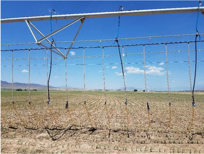
Figure 3. The filters can be seen on the feed lines from the pivot pipe above. Whole system filtration near the pump is recommended if the entire pivot uses MDI. The ties used to keep the rigid drops vertical can also be seen secured to the truss rods. Photo by Troy Peters.
