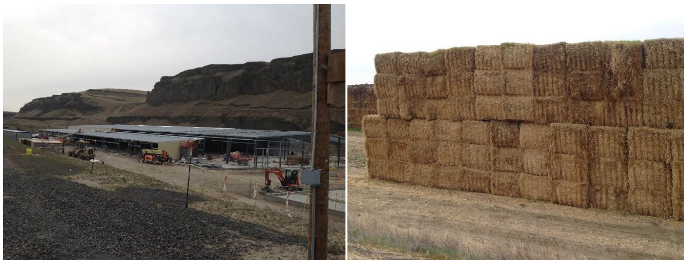
Figure 7. Pulp mill processing plant under construction near Starbuck, WA (left). Wheat straw bales stored near the construction site (right). Photos taken April 3, 2018 by W. Pan.
