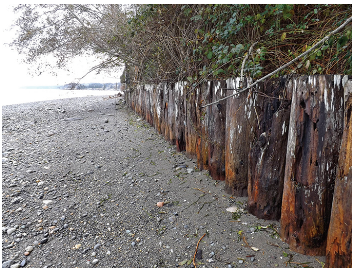
Figure 22. Eroding wood bulkhead. Photo by Scott Chase.
