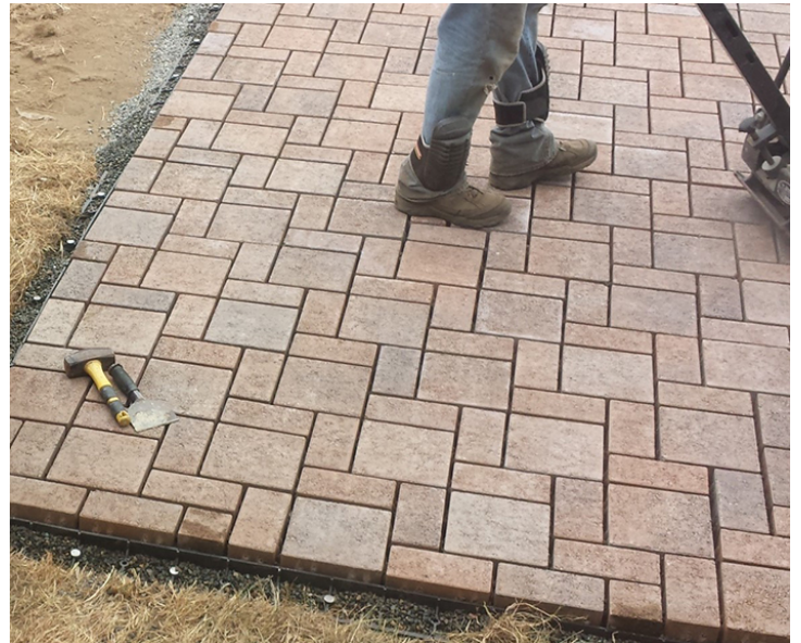
Figure 20. Installing permeable pavers allows water to flow into the ground via the cracks. Photo by Scott Chase.
