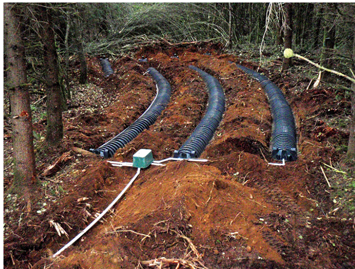
Figure 4. Drainfield pipes are not buried very deep. Photo by Alan Chapin.
