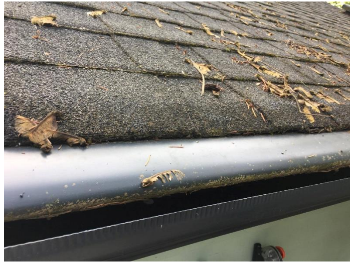
Figure 3. Gutter guards prevent the accumulation of biological debris in the gutters and rain barrels. Photo: D.Y. Leggett.
