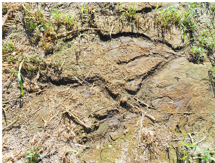
Figure 3: Early channelization forming in a bare spot within a VFS. (Photo by B. Bodah)
