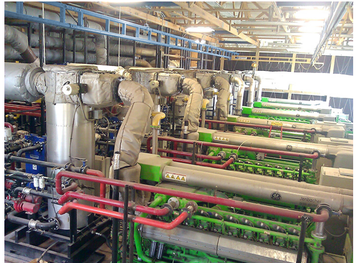
Figure 5. Three engine and generator sets were added at a co-digestion facility to handle additional biogas production from substrates; the new total output doubled to 6.3 megawatts. (Photo courtesy of DVO, Inc.)
