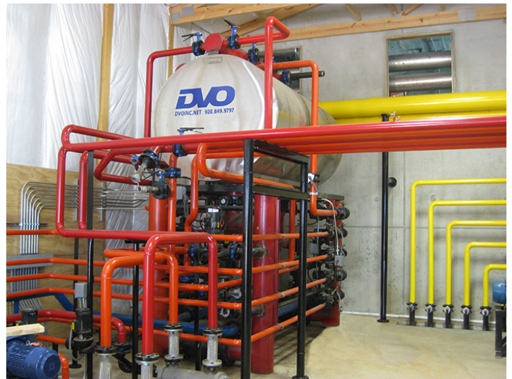
Figure 9. Operating costs include maintaining and monitoring equipment to minimize digester failures and inefficiencies. Color-coding of piping helps workers quickly distinguish biogas (yellow) from water (orange, red, and blue). (Photo courtesy of DVO, Inc.)
