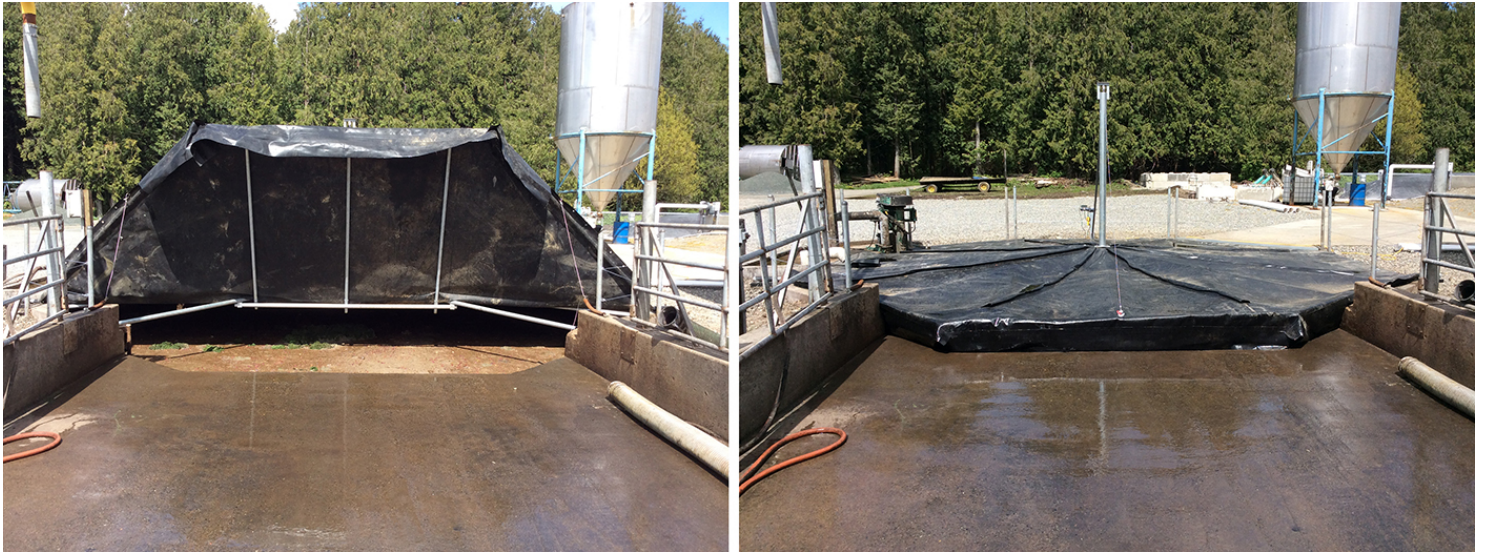
Figure 4. Automated covers, placed on top of receiving pits, can be opened for substrate addition (left) and closed to minimize odor release (right). (Photos courtesy of Andgar Corporation.)
