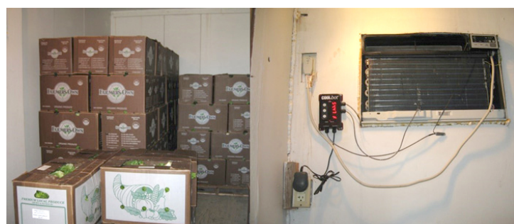
Figure 38. A homemade cold room for salad crops, maintained at 32°F and 95–100% humidity, using an air conditioner and temperature-control unit.
