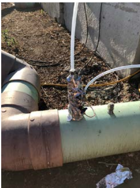
Figure 6: Ejector diluter on the negative aeration duct. Smaller diameter tubing is the zero air supply from the van. Larger ID tubing extending vertically is the sample air flow out to the van instrumentation. Wires seen at the bottom of the ejector diluter power resistive heating wires heating the body and the 1/16-in sample tube projecting into the duct.
